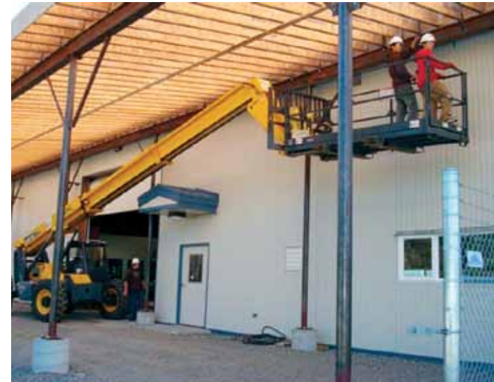
DGSD high school CT students help construct the new sidewalk and headbolt heaters (above left) and covered storage (above). CT students benefited from hands-on learning during the semester and some were hired as a summer crew to help complete the projects funded by a Rasmuson Foundation grant.
