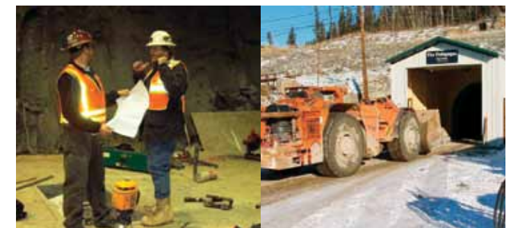
Left: DMTC Executive Director Whit Hicks (right) discusses the plans for the new underground control room with employee Jeb Timm. Right: A Scoop Tram Toro 007 enters the portal to the underground mine. The Scoop is used to muck out the mine after blasting. DMTC operates an underground training mine.
